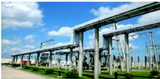
Zhoushan DC Transmission Converter Station
