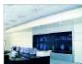
Jiang Chong Power Automation System Shanghai Province
