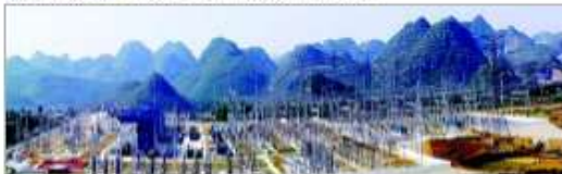
Guihou-Guizhou 1 (500KV DC Power Transmission System) Guizhou Province
