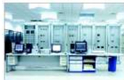
CCZ-8000 Thermal Power Plant Automation System
