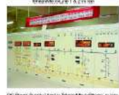
DC Power Supply Used in Sheng Metro Project in Iran
