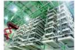
Dushou Converter Station 1 200KV HVDC Power Transmission System
