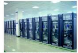
Siemens Control Cabinet Workshop
