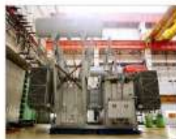
220kV Power Transformer
