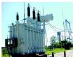
110kV Oil-immersed Power Transformer
