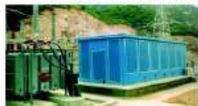
35KV Outdoor Prefabricated Substation Shanghai County, Henan Province, China
