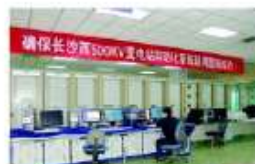
CCZ-8000 Substation Automation System
