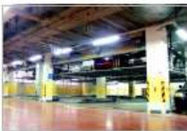
Shahin Shopping Mall Phase II Apartment Car Parking System
