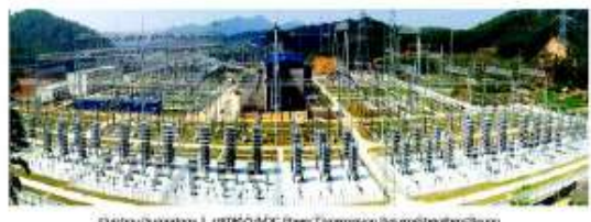
Dushou Converter Station 3 200KV HVDC Power Transmission System
