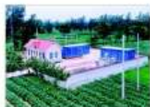
25kV Outdoor Prefabricated Substation Shanghai County, Henan Province, China
